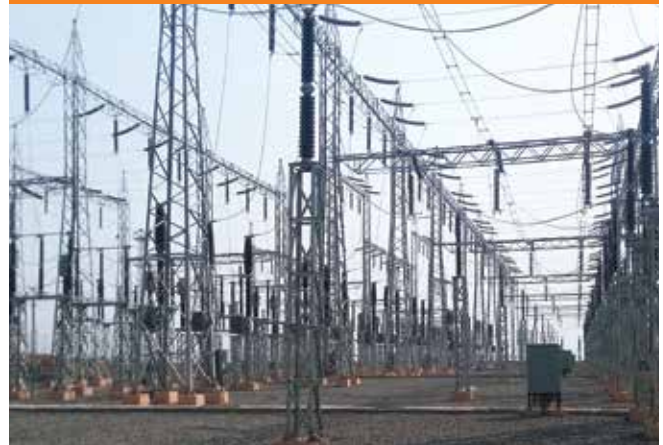
220 kV AIS Sub-Station for MSETCL
