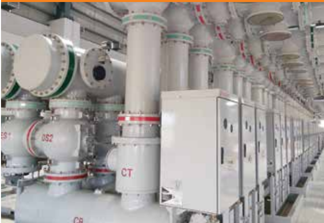
400 kV GIS Sub-Station for GETCO
