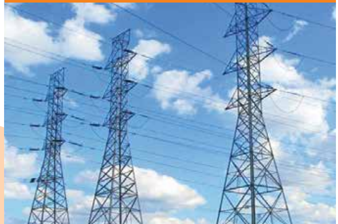
220 kV Transmission Line for MSETCL
